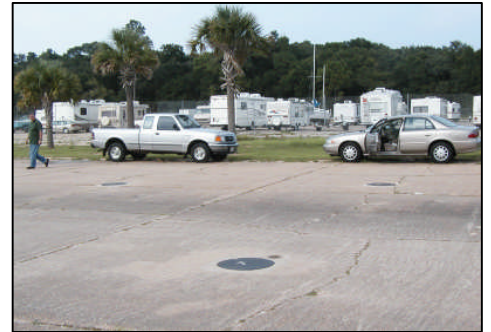
Figure 1: Site 1140MW at OLF Bronson, NAS Pensacola, FL.
